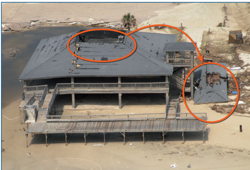
FIGURE 2-2: Roof structure failure on a house (Galveston, TX, 2008) (SOURCE: FEMA P-757)
